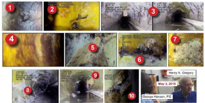
(Below) Henry Gregory reviews CCTV and FELL technologies on a failed West Coast CIPP lining project (2016).
