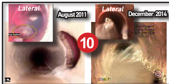
10. Misreported Bad Reconnection. Same Leak Running 4 Years.
