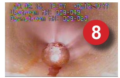
8. Unreported Contractor Damage
