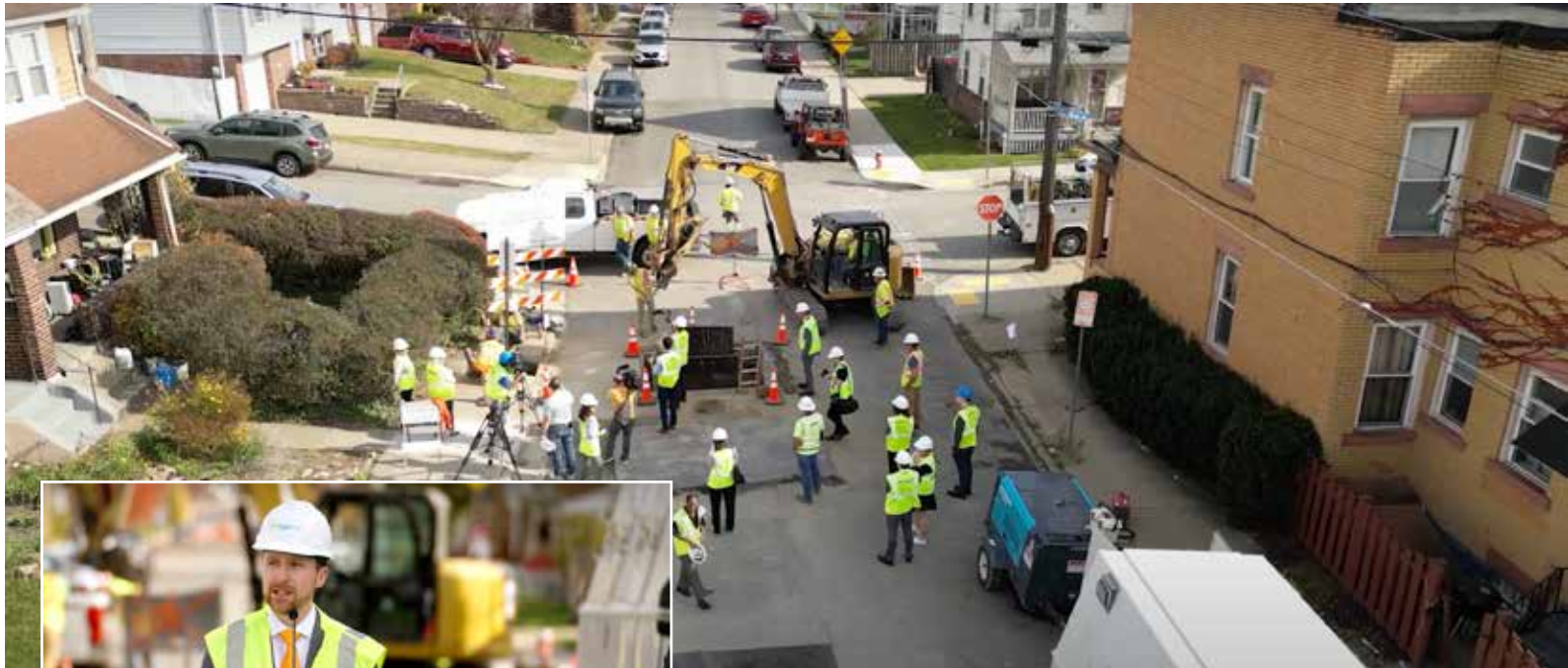
(Left) Will Pickering, CEO, Pittsburgh Water, speaking at an event celebrating the removal of PGH20's 12,000 th lead water pipe. On track to eliminate all lead water service lines by 2027.
