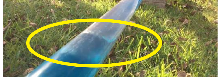
Figure 40. Baseline Disturbance from Re-Energizing Water Services.
