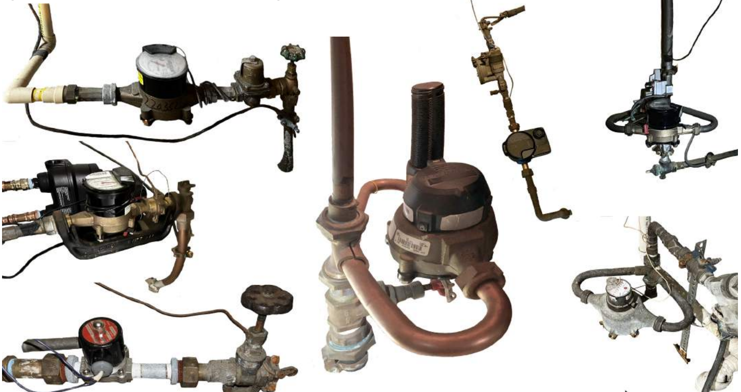
Figure 29. Various Basement Meters and Service Configurations.
