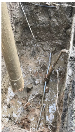
Figure 4-1. Application of the Potholing Technique for LSL Exposure at the Curb Stop.
