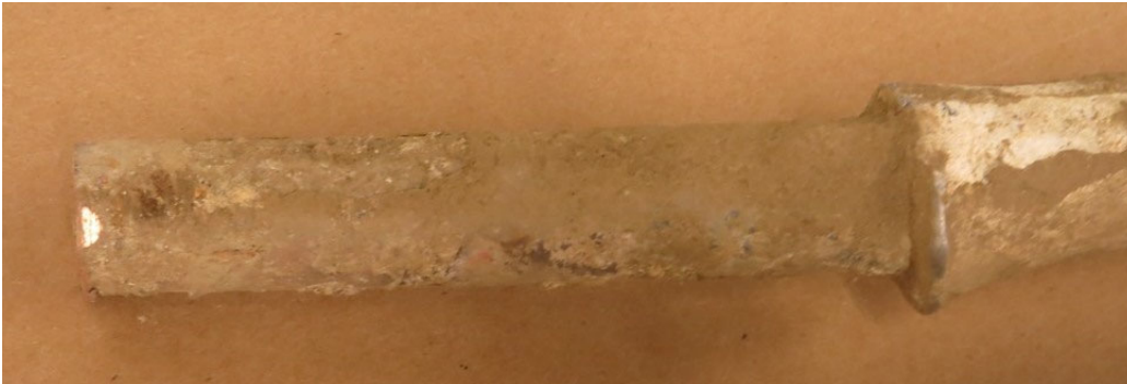
Figure A-11. Coupling between Lead and Copper Pipe – Sample 16-0209-CP-2 Side A.
