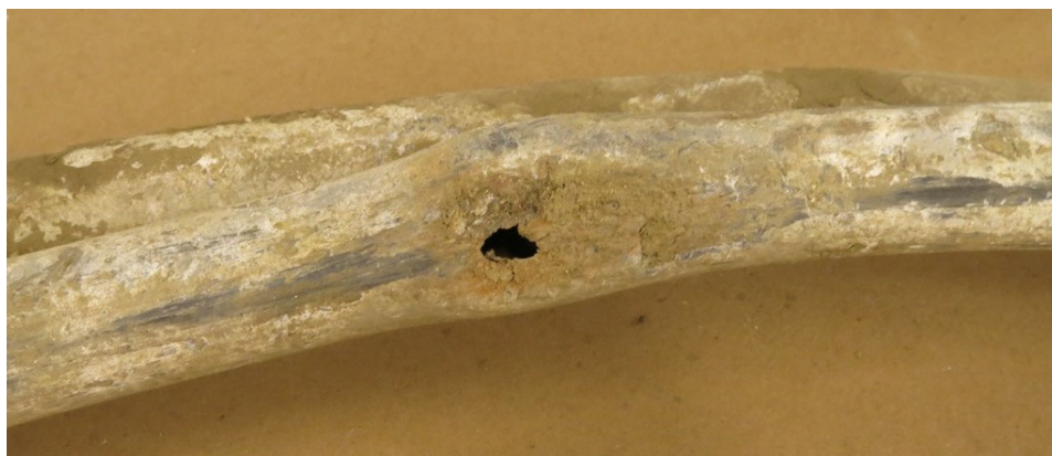
Figure A-18. Hole in the Lead Pipe from Sample 16-0209-CP-2.
