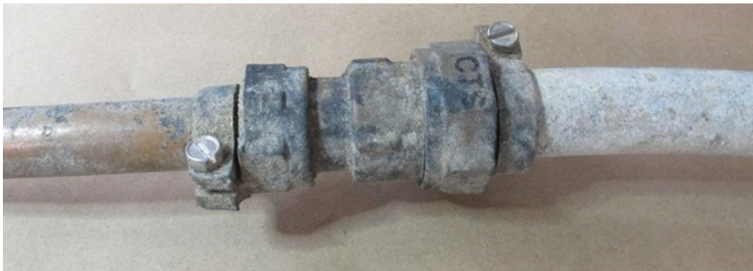
Figure A-12. Coupling between Lead and Copper Pipe – Sample 16-0209-CP-4.
