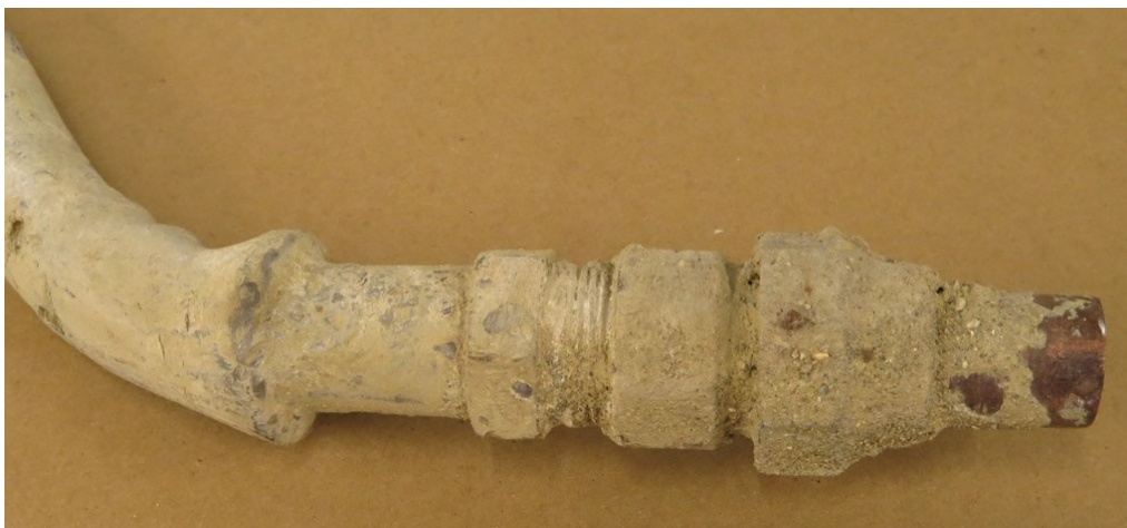
Figure A-9. Coupling between Lead and Copper Pipes – Sample 16-0209-CP-1 Side A.
