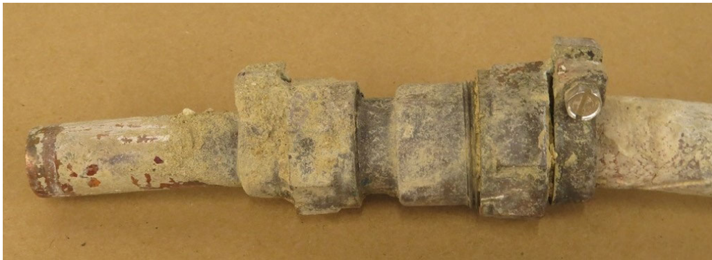
Figure A-10. Coupling between Lead and Copper Pipes – Sample 16-0209-CP-1 Side B.
