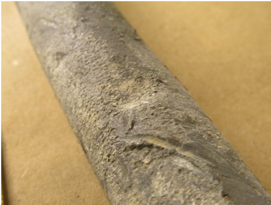
Figure A-14. Damages on the Surface of a Lead Pipe from Sample 16-0209-Pb-1.
