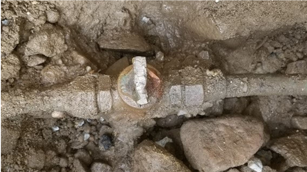
Figure 4-4. Curb Stop Valve at Location 6.
