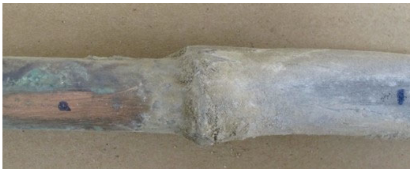
Figure A-13. Coupling between Lead and Copper Pipe – Sample 16-0209-CP-5.
